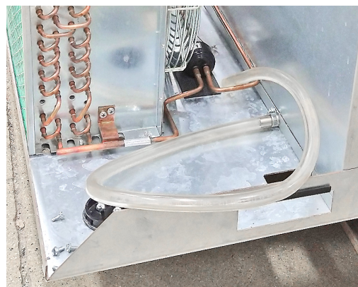
Ice-Bank Overflow-Drain Hose (from Standpipe)
